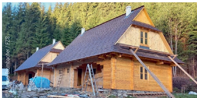
New high quality and ecological ranger houses constructed in accordance with traditional architectural practices were built in Ukraine's Verkhovynskiy National Nature Park, near the Romanian border. A second building functions as a guesthouse for tourists.
